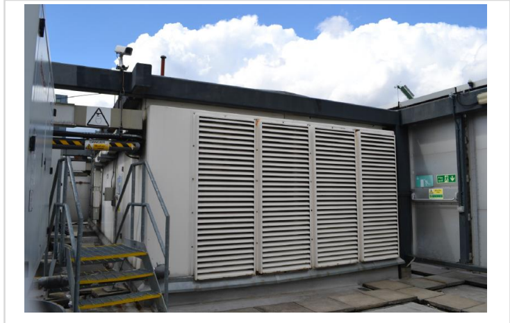
Protected UPS Generator Room
